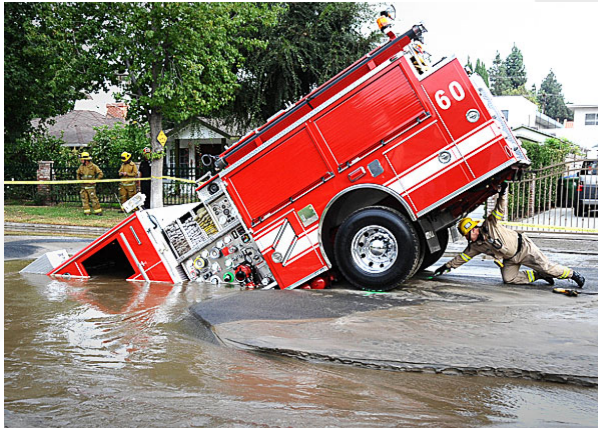
Water Main Failure, Los Angeles 2009
